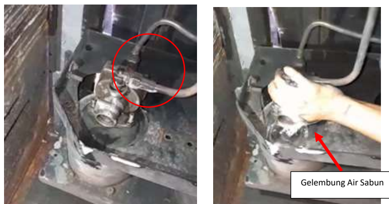
Gambar 14. Kondisi exhaust relay valve
