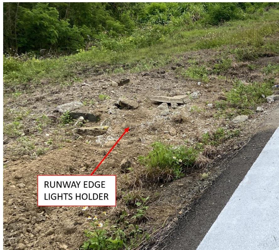
Figure 3: The damage of runway edge lights
