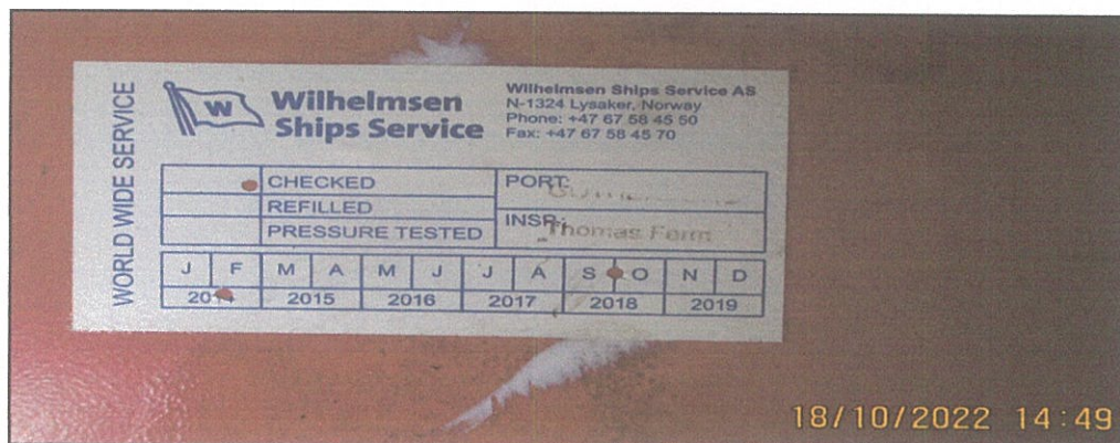
Gambar I-29: Pengecekan terakhir release cabinet Sistem CO2
